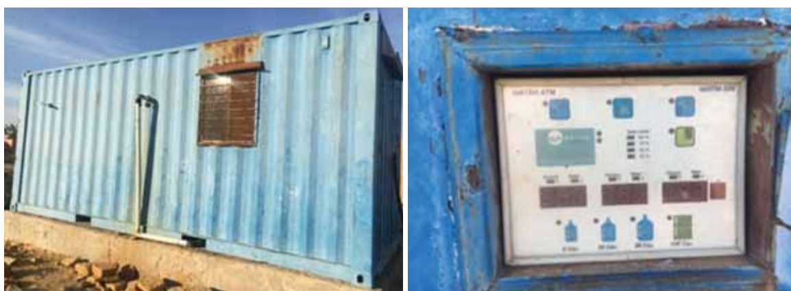
Figure 12: Water treatment plant at Dedha village
